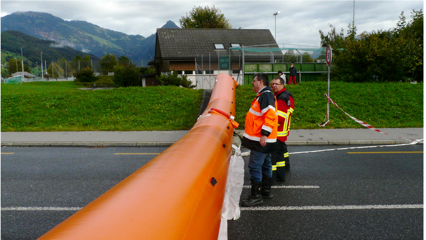
Einsatzbereiter Beaver (2011) An inflatable Beaver barrier installed for a flood event (in 2011),
